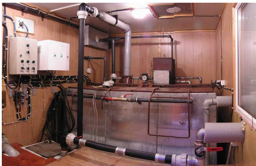
Figure 3. Facility for treatment of sewage waters at Progress station
